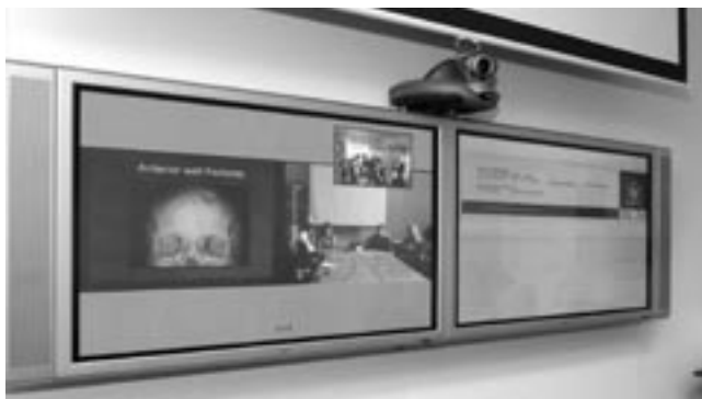
Video Conferencing Facility installed in Radiology Tutorial room in RCSI.
